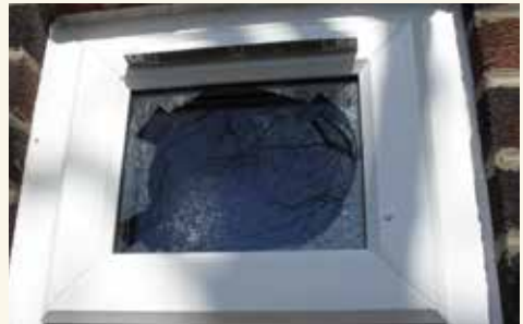
✗ Not acceptable standards
