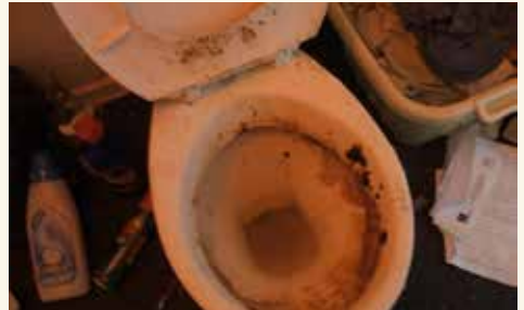
✗ Not acceptable standards
